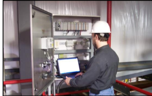
ECT provides full field service support, from checkout to commissioning and remote support for system troubleshooting.
