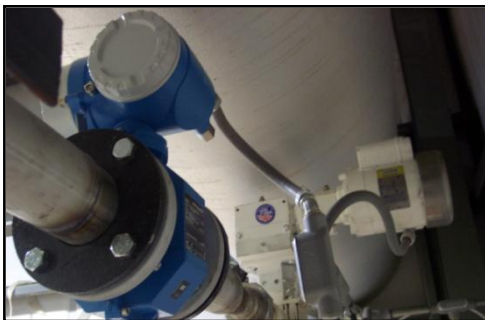
ECT's engineers review field-mounted devices for optimum control system performance.
