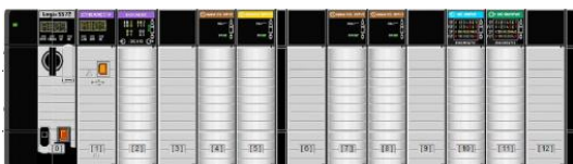
ECT's FuelPAC Turbine Control System Using Standard Rockwell Automation Hardware and Software
