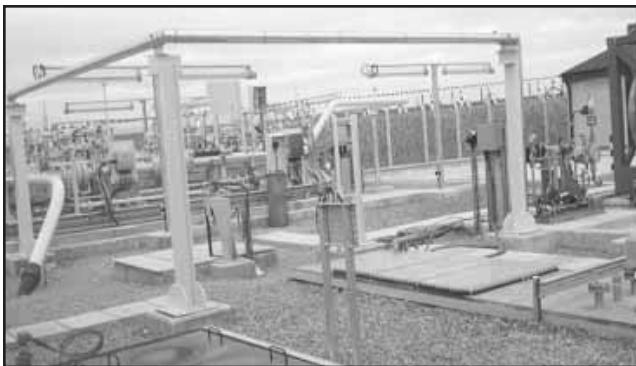
Monitoring water discharge from covered separators in unmanned locations
