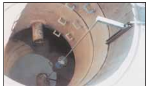
Leakwise ID-223 installed in a sump collecting water from a separator at a pipeline pumping station
